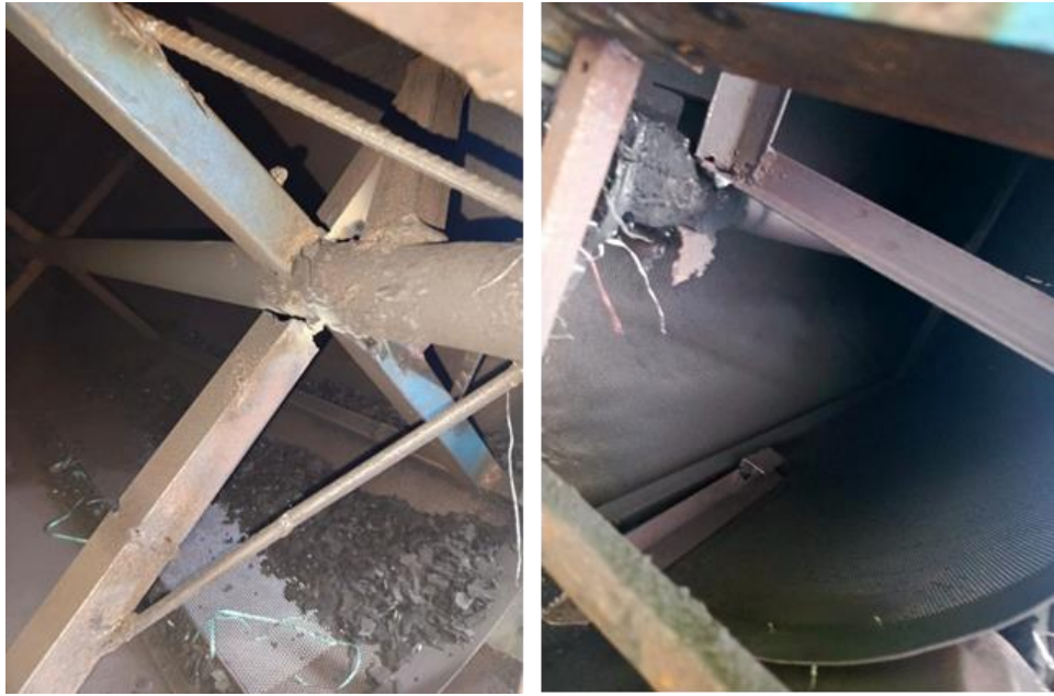
Figure 3. 1 Condition of the broken shaft support before replacement
