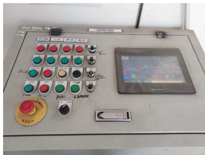
Gambar 6. Panel box operator conveyor
