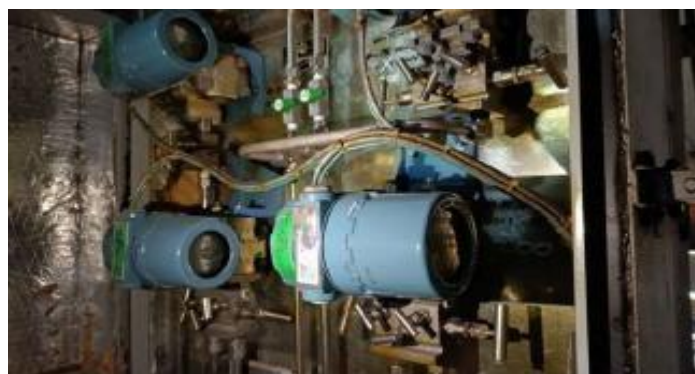
Gambar 7. Sensor Pressure Transmitter
