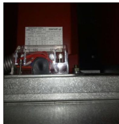
Gambar 10. Name Plate pada CT (Current Transformer)
